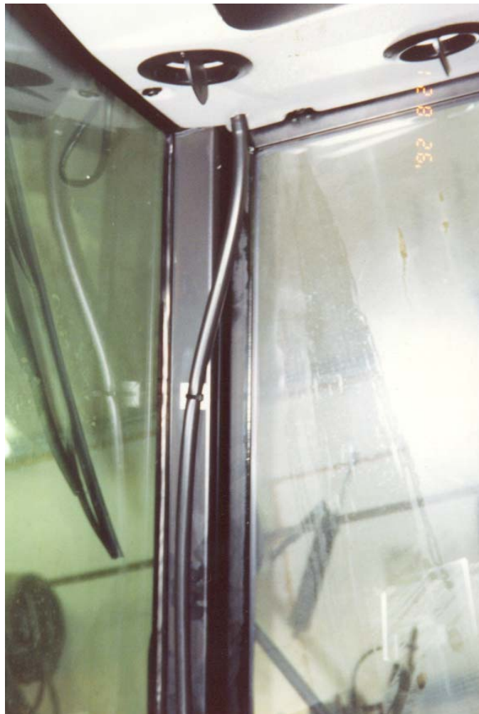
Showing drain tube coming through roof.
